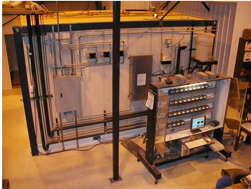
Figure Error! Style not defined.-2: Climate chamber test facility
