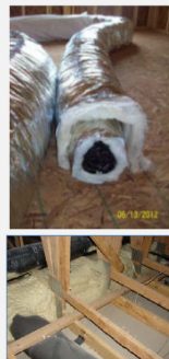
Compact Buried Ducts in a Hot-Humid Climate House - HIRL 2016
