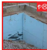
A. Slab insulation does not extend to the top of the slab.
