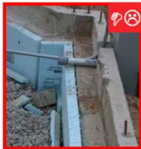
A. Slab insulation does not extend to the top of the slab.
